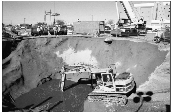
54-inch Diameter Sewer Collapse
