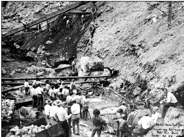
Crews lowered the first stone at Roosevelt Dam on September 20, 1906. This cornerstone sits on the bedrock of the Salt River and established a firm footing for the Salt River Project.
