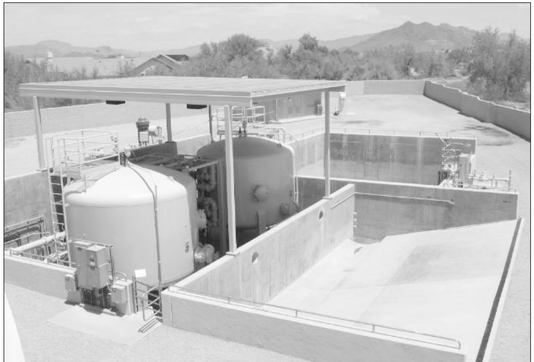
Arsenic Treatment Facility at Well 280
