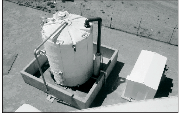
Brine Handling Facilities
