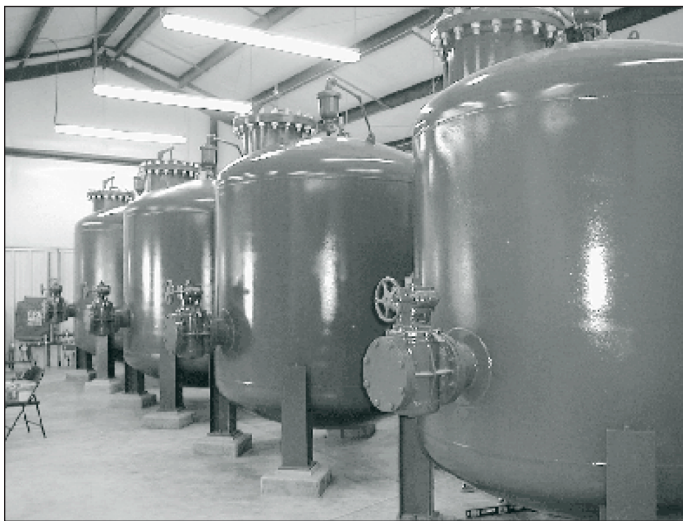
Ion Exchange Treatment Vessels
