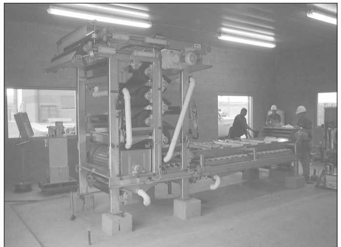
Sludge dewatering belt press
